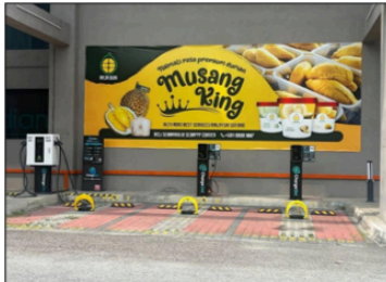
EV charging stations
