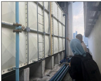
Rainwater harvesting system
